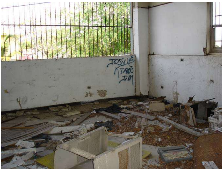
Picture 31. Accumulation of debris inside main structure.
