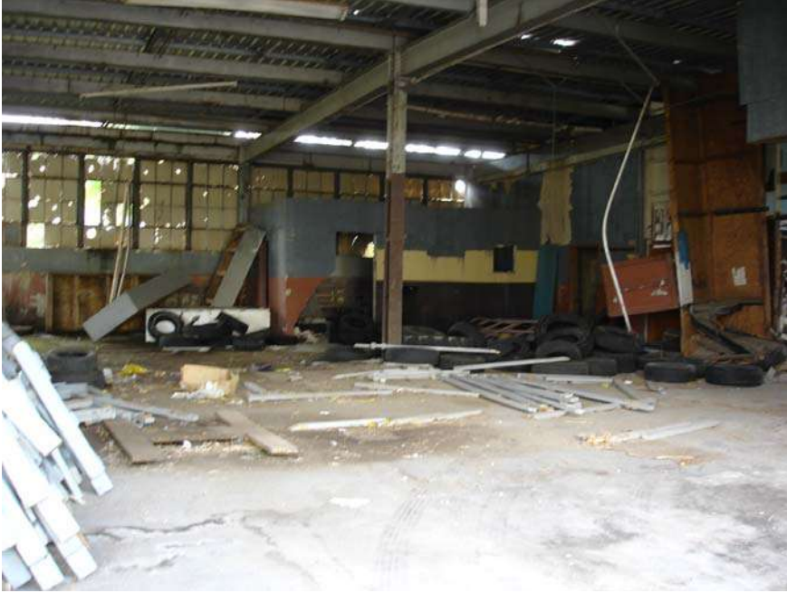
Picture 32. Accumulation of waste inside main structure.
