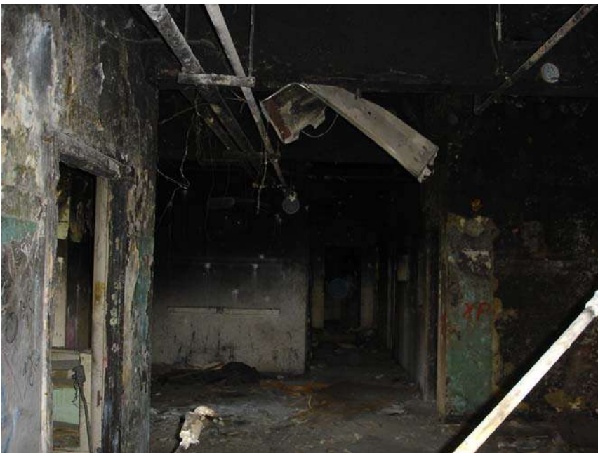
Picture 79. Structure showed signs of fire damage.
