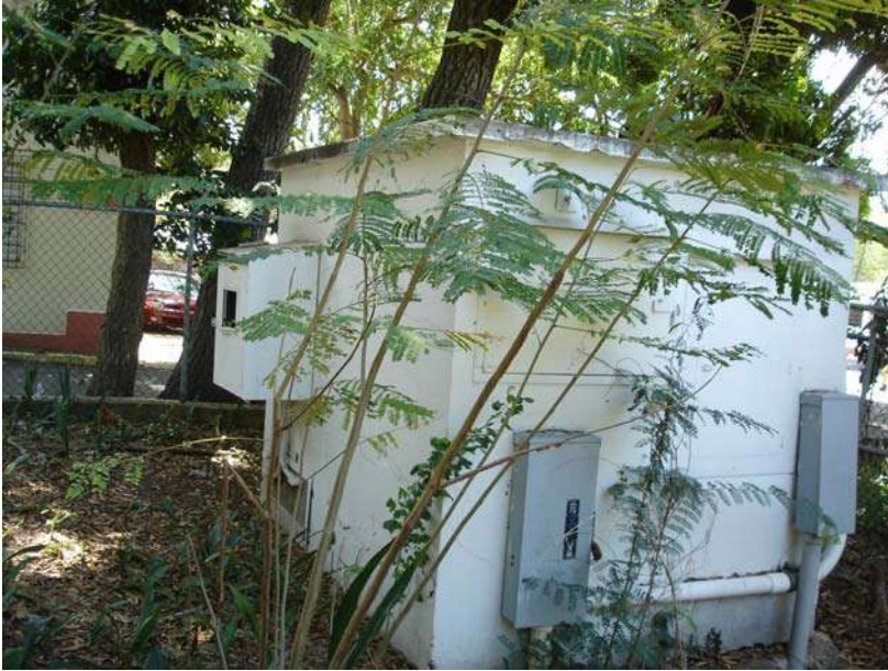
Picture 113. An electrical substation was also located at this parcel.
