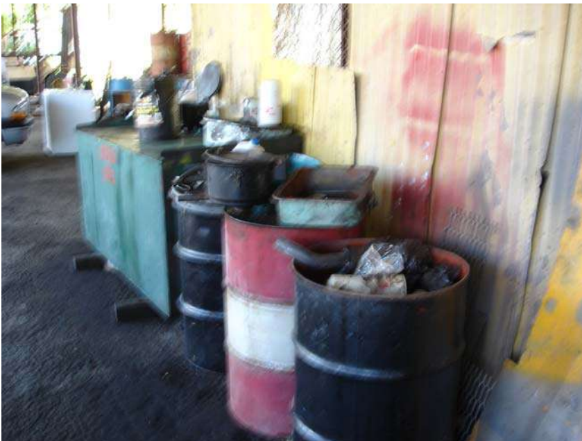
Picture 57. Stained concrete floor.
