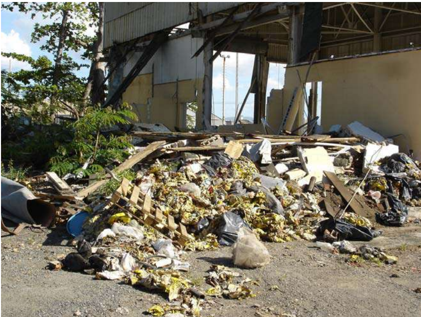
Picture 102. Debris generated and accumulated at this location.
