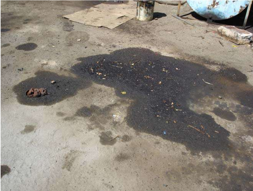
Picture 64. Stained concrete surface.
