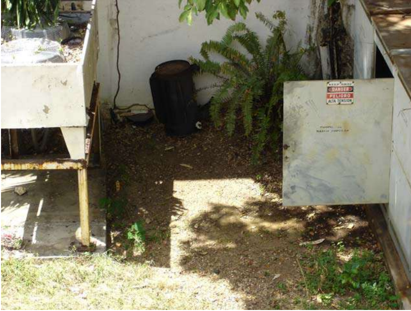
Picture 92. Abandoned electrical sub-station west of the main structure.
