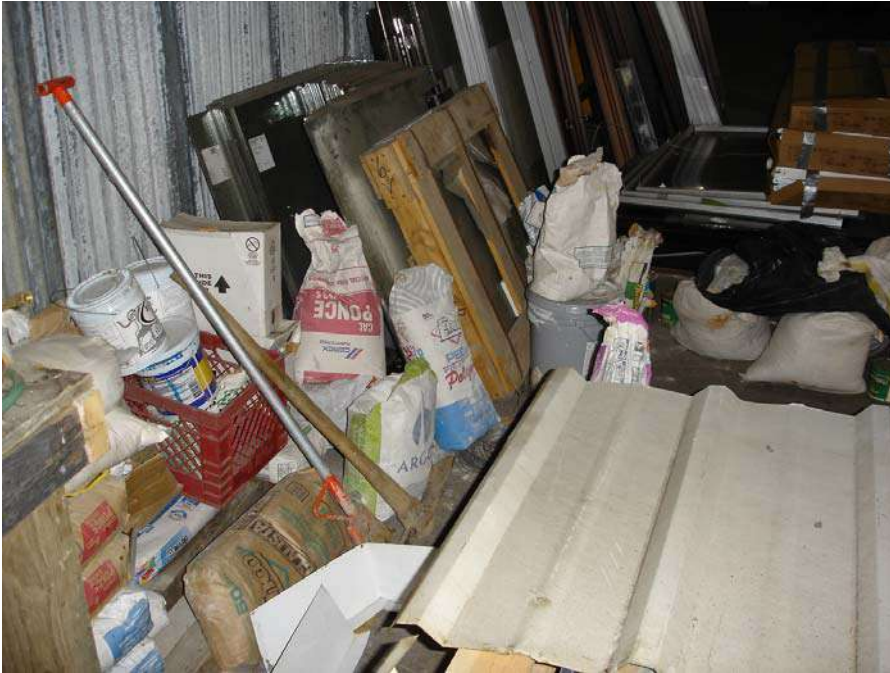
Picture 21. Construction and paint-related material storage inside the main building.
