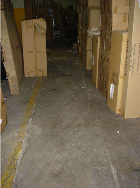
Picture 15. Underground drainage system covered by concrete slabs.
