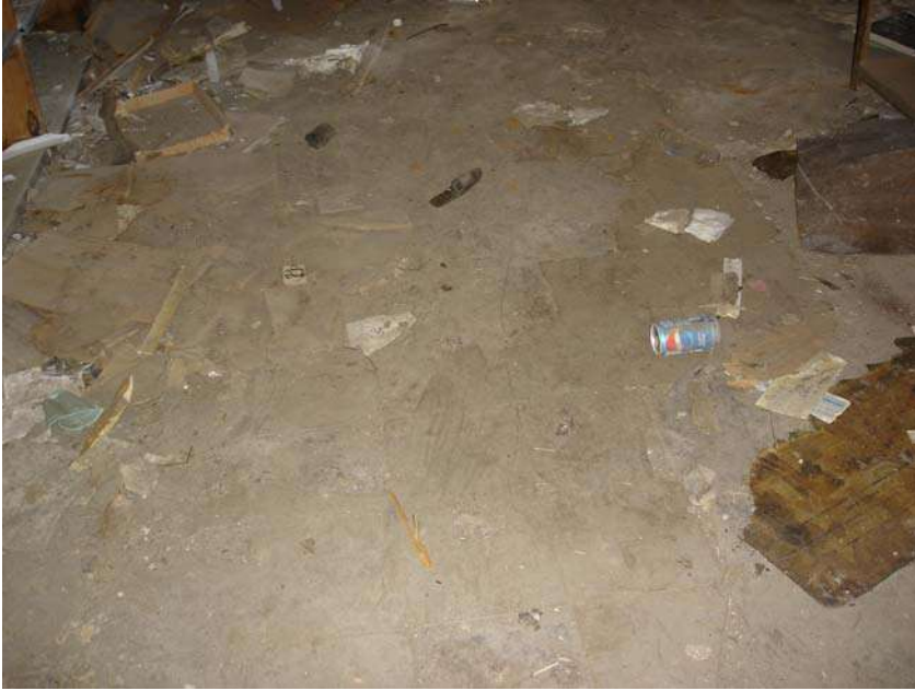
Picture 84. Vinyl tiles at the main structure may contain ACMs.
