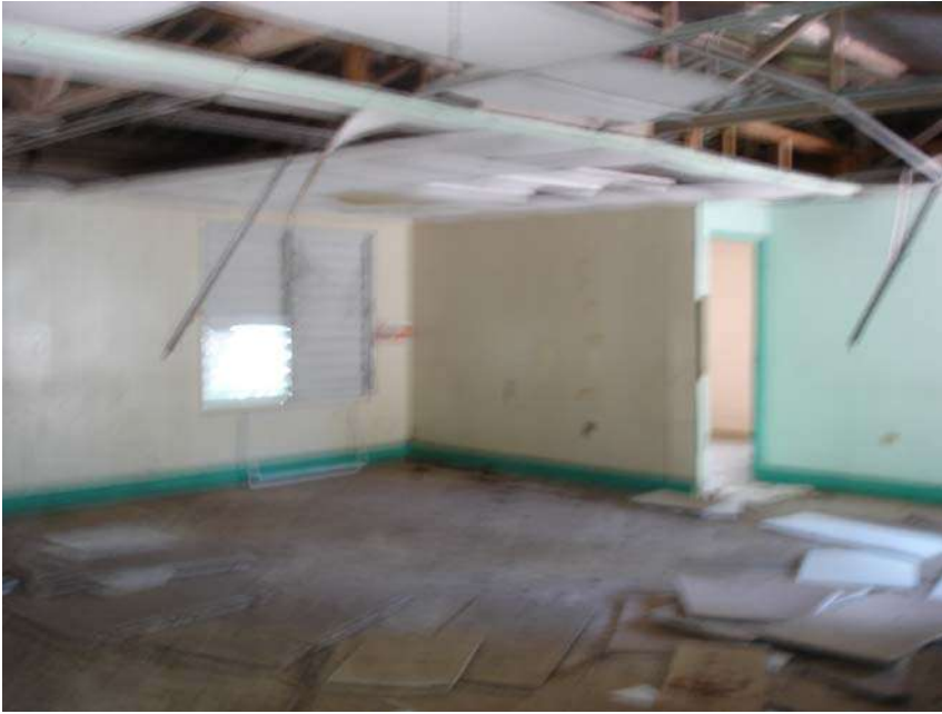
Picture 111. Floor and ceiling materials may contain ACMs.
