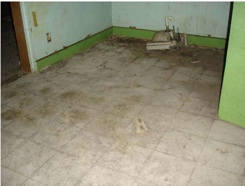
Picture 121. Floor tiles may contain ACMs.
