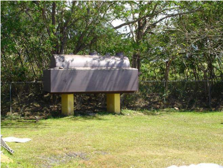
Picture 122. Double-walled AST documented at the site.
