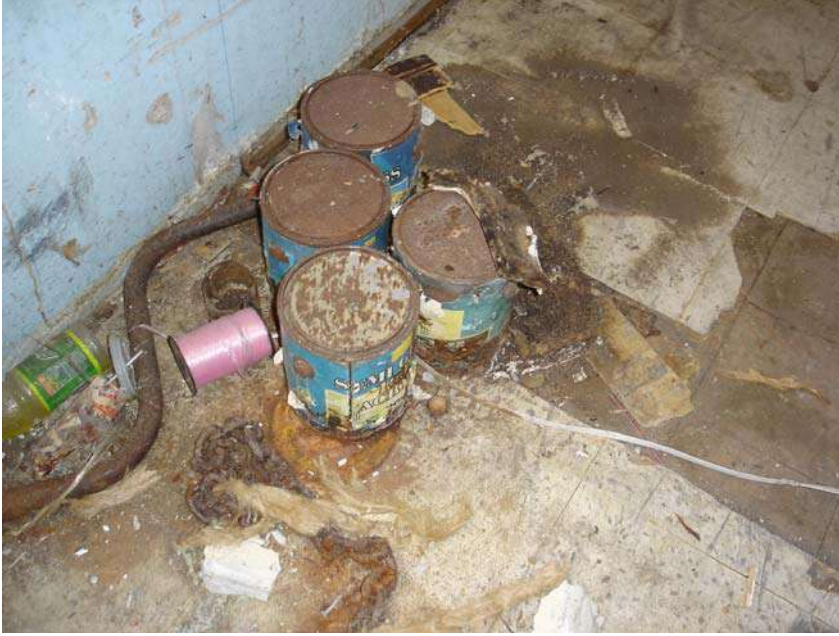
Picture 88. Accumulation of paint related products inside the main structure.
