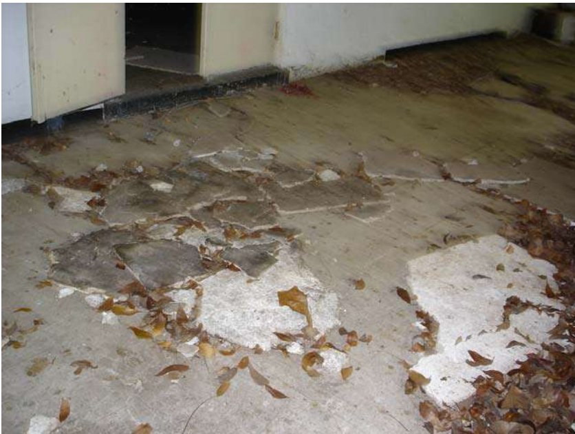
Picture 119. Floor tiles may contain ACMs.
