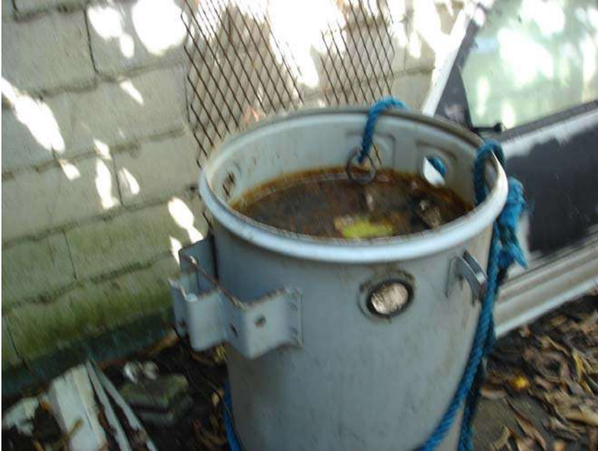
Picture 54. Electric transformer full of what appears to be dielectric oil.
