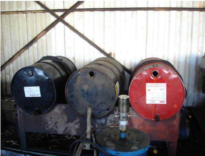
Picture 55. Oil and lubricant dispensing station.
