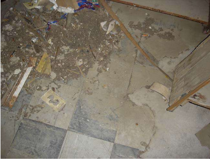
Picture 82. Vinyl floor may contain ACMs.
