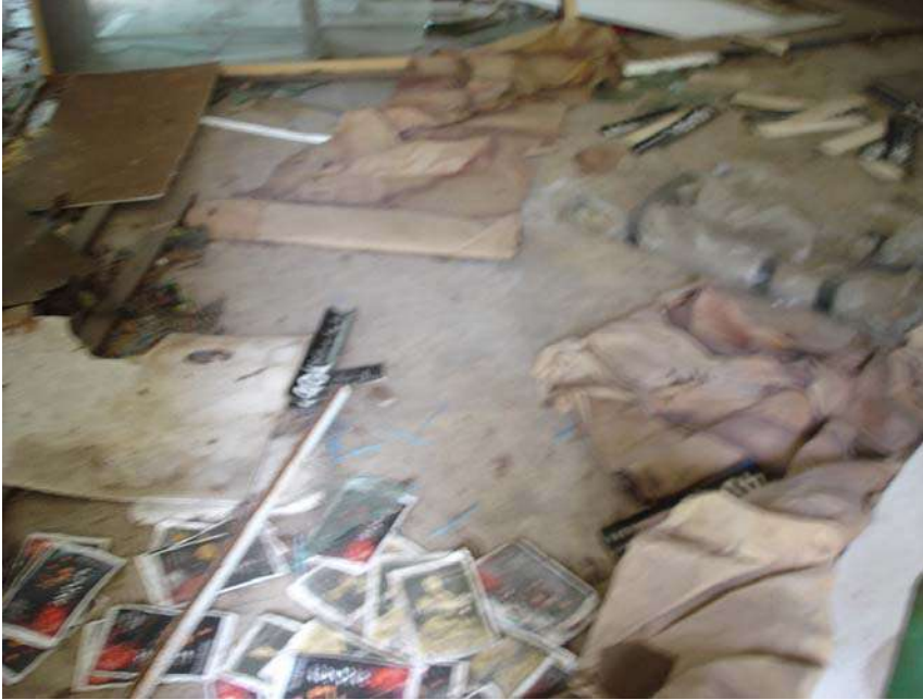
Picture 116. Accumulation of debris at one of the structures.
