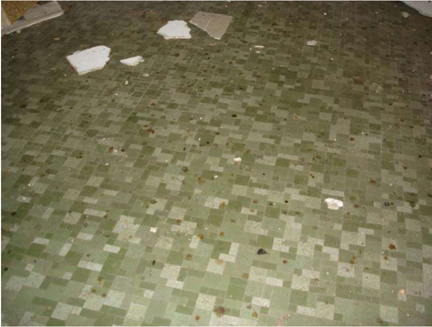
Picture 118. Floor tiles may contain traces of lead.
