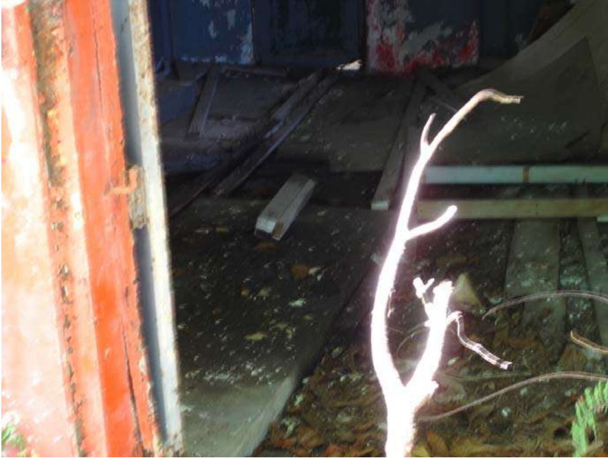
Picture 6. Evidence of oil stains on a floor section of the structure.
